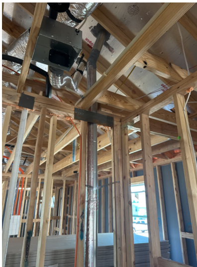
VENTS TO ROOF
