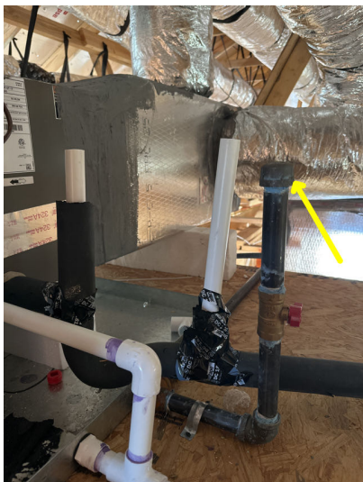
GAS SUPPLY CAPPED
