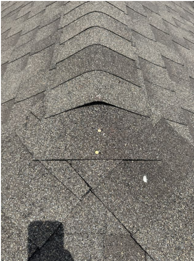
FASTENERS NOT SEALED
