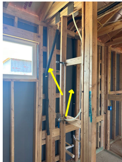
SUPPLY LINES INSULATED
