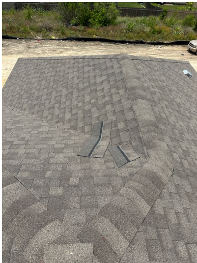
DEBRIS ON ROOF
