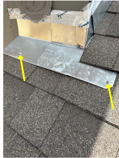
FASTENERS NOT SEALED
