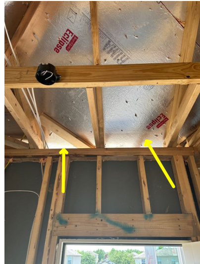
GAPS AND CRACKS BETWEEN WALL AND EAVE
