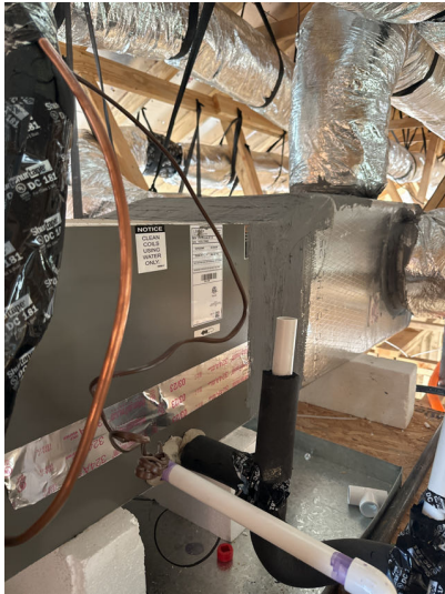
AIR HANDLER PROFESSIONALLY INSTALLED
