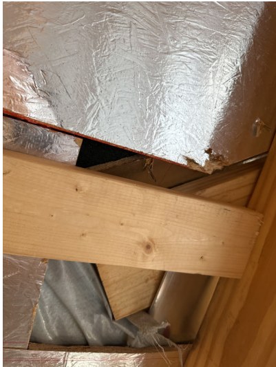
DECKING ISSUES ABOVE GARAGE
