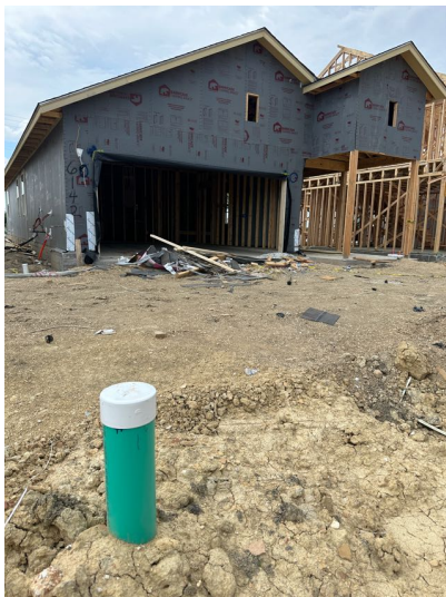
STREET SIDE CLEANOUT
