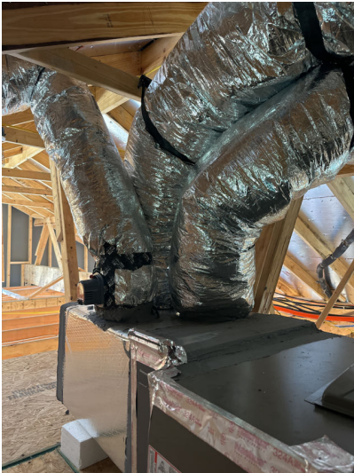
DUCTING PROPERLY SUPPORTED
