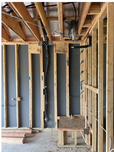
STAGED FOR INSTALLATION
