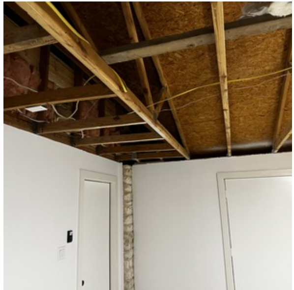
GARAGE: MISSING FIREWALLS
