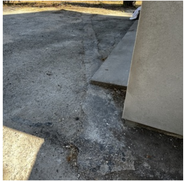
CUT/PATCH: PREVIOUS PIPE REPAIR
