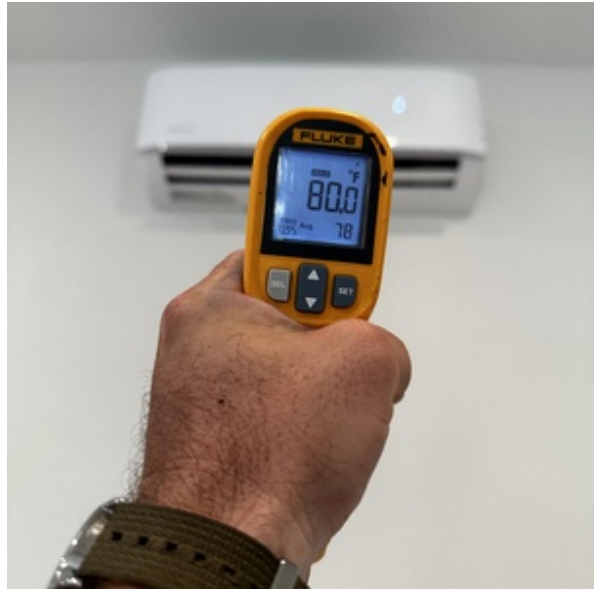
MINI-SPLIT FAILED TO COOL
