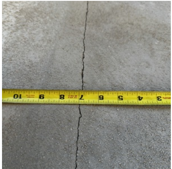
CRACKS AT RECENTLY INSTALLED CLADDING
