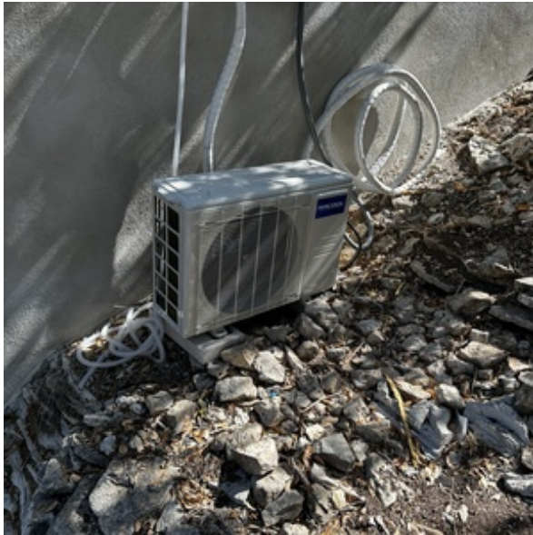
INSTALLATION AND FUNCTIONALITY ISSUES
