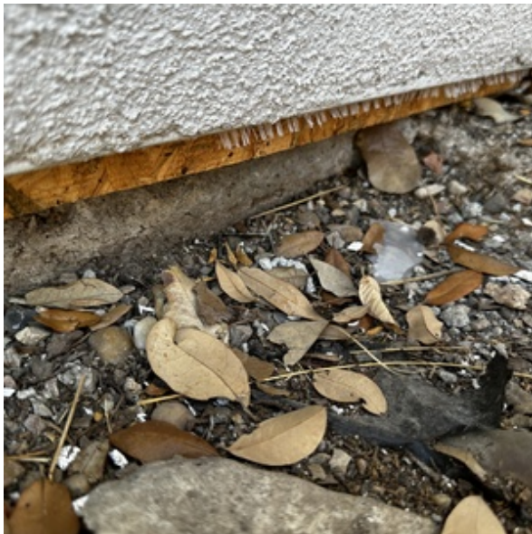
EXPOSED PLYWOOD UNDER STUCCO
