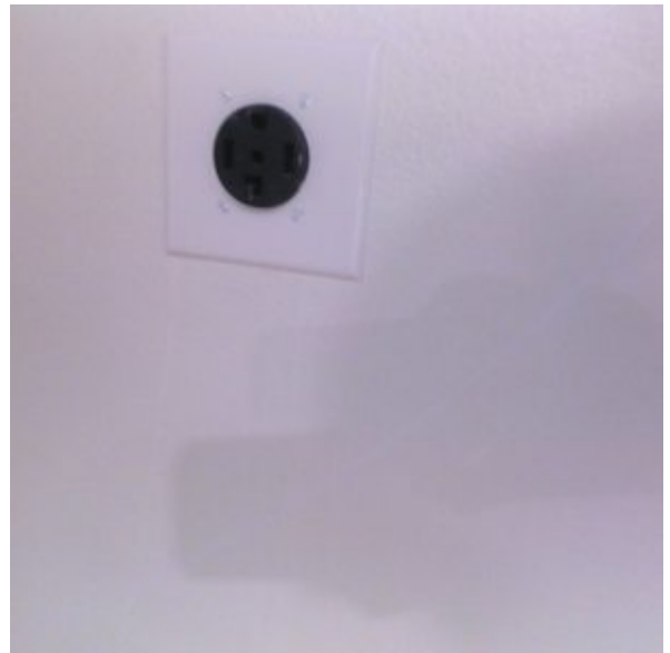
LEAK EXITING AT DRYER OUTLET
