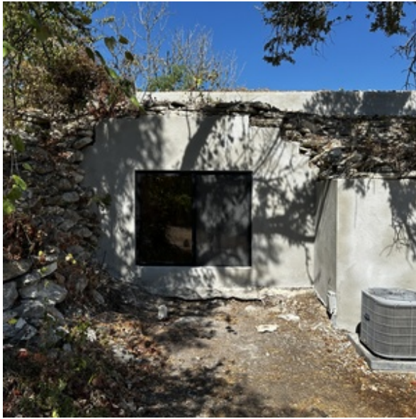
DRAINAGE CONCERN OVER WINDOW
