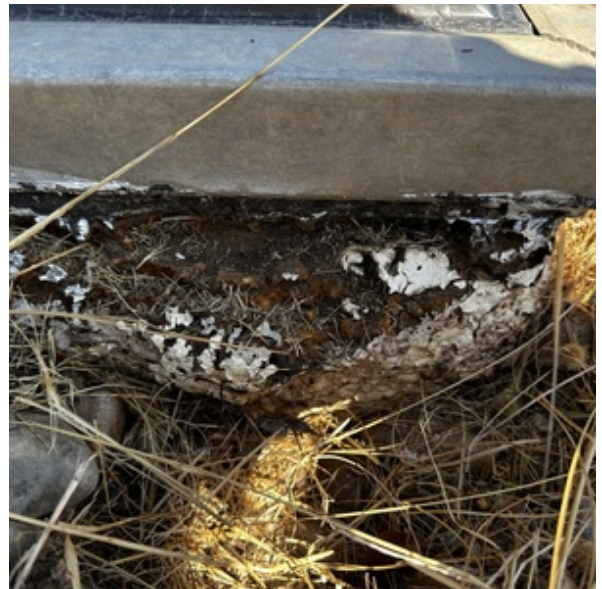
DETERIORATION OF FOAM SURROUNDING
