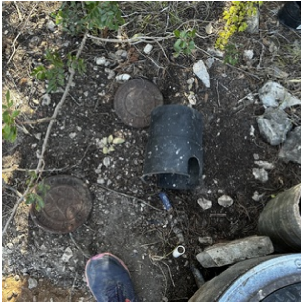
WATER METER RIGHT OF BLDG.
