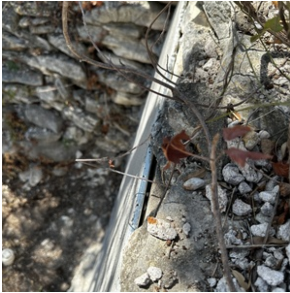
NO UPPER CLADDING FLASHING
