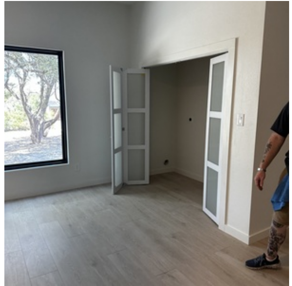
LEAK DISCOVERED IN LAUNDRY
