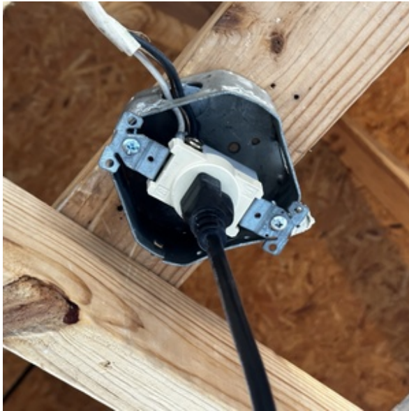
MISSING SAFETY PLATES
