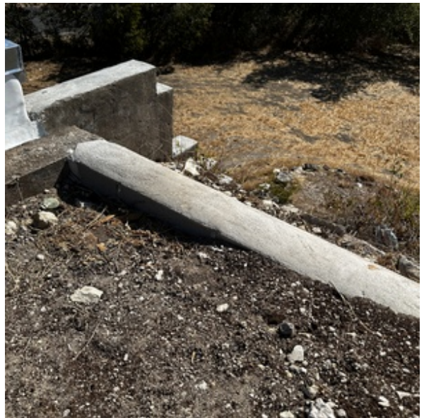
DRAINAGE PATH CONCERNS
