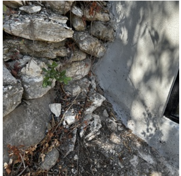
LOOSE DRY STACK ABUTTING WALLS
