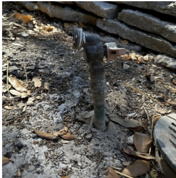
PROTECT PIPE, ADD ANTI-SIPHON
