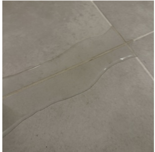
LEAK AT BEDROOM SINK
