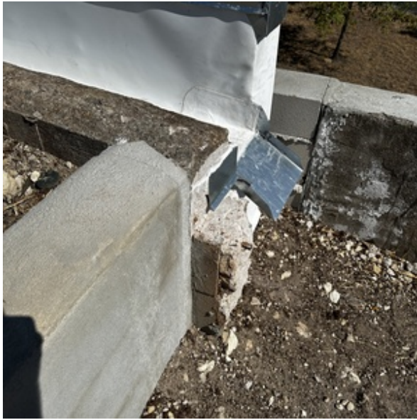
ROOF INTERSECTION CONCERNS
