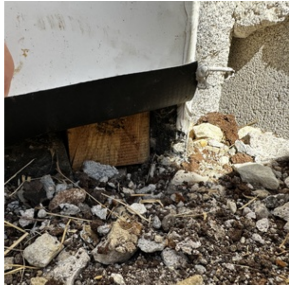
EXPOSED PLYWOOD, LOOSE TPO
