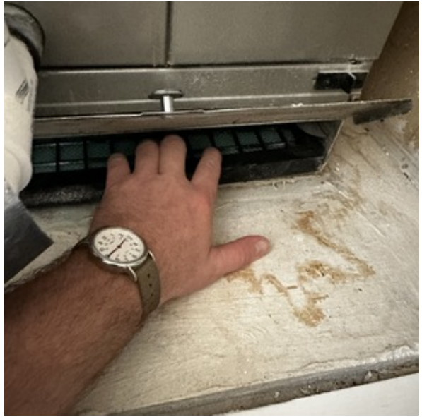
PREVIOUS HVAC LEAK
