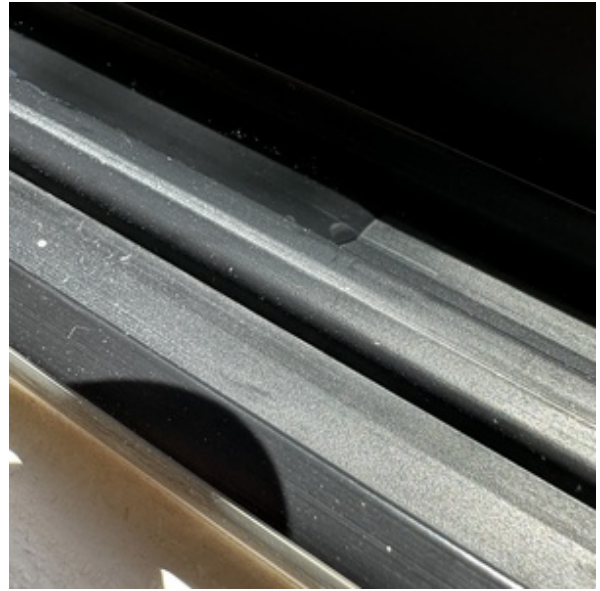
WATER FILLS WINDOW SLIDE WELL
