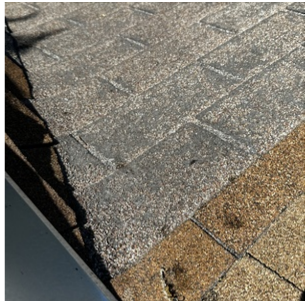
REMAINING SHINGLES IN POOR CONDITION
