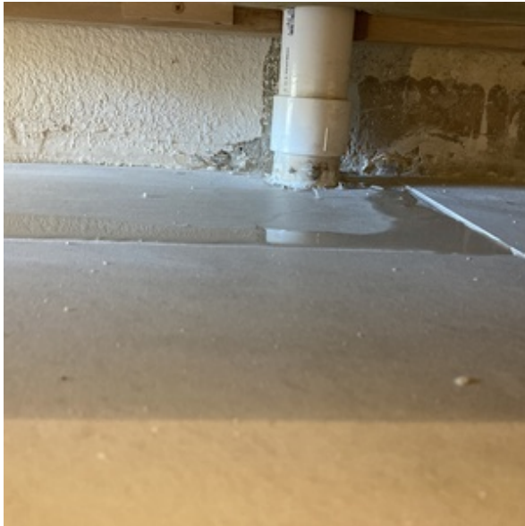
LEAK UNDER BATHROOM SINK
