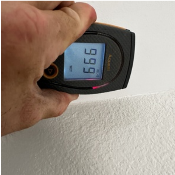
DINING: ELEVATED MOISTURE READINGS
