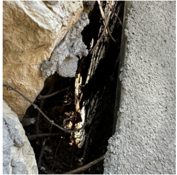
ATYPICAL DRAINAGE POINT AT STONE/CLADDING
