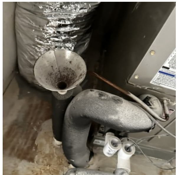
MYLAR FLEX DUCTING OBSERVED
