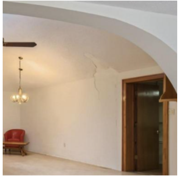
PREVIOUS DAMAGE NEAR HIGH READING
