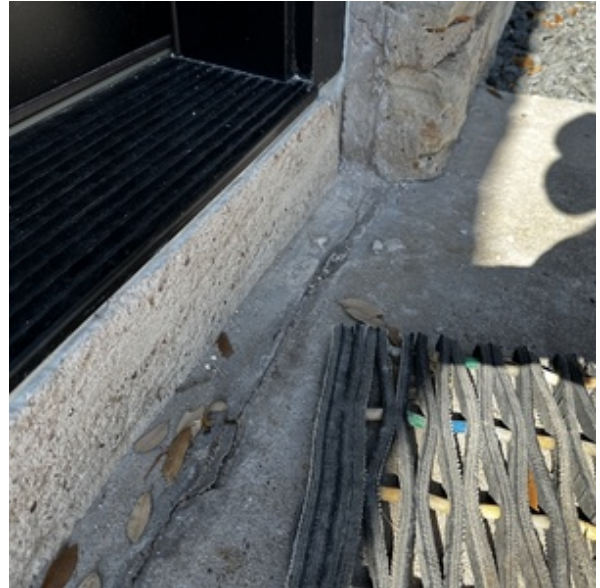
CRACKS AT ENTRY PORCH/LANDING
