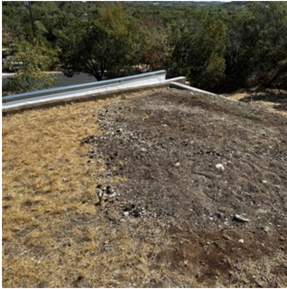
AREA OF PREVIOUS REPAIR
