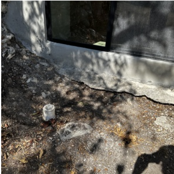
DRAINAGE ISSUE NEAR LEFT WALL
