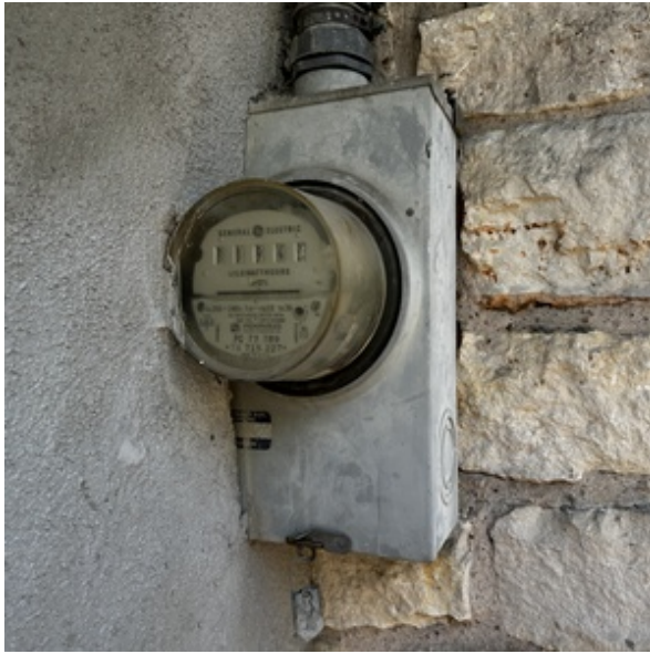
DATED METER CAN PARTIALLY COVERED
