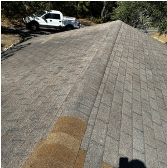
REMAINING SHINGLES IN POOR CONDITION
