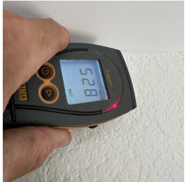
DINING: ELEVATED MOISTURE READINGS
