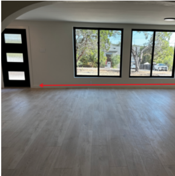
VISIBLE UNEVEN FLOOR SURFACE
