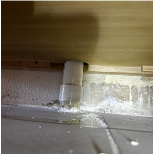
LEAK AT BEDROOM SINK
