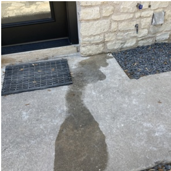
LEAK OVER LAUNDRY/NEAR MAIN ENTRY
