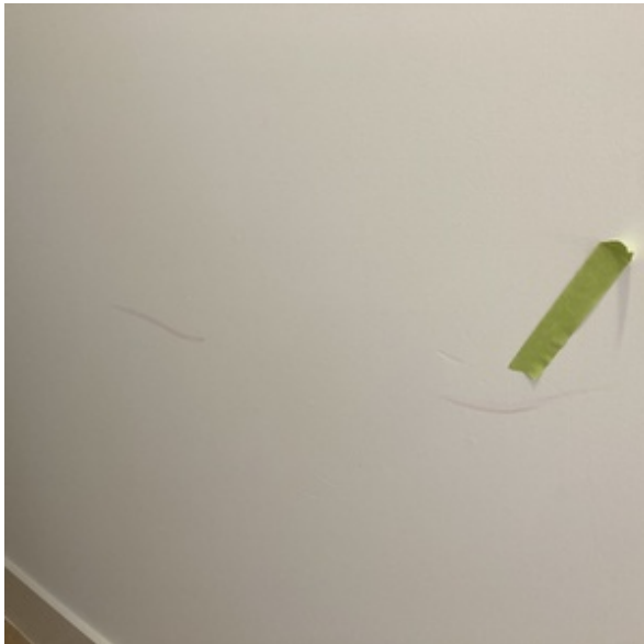
MINOR FLAWS MARKED ON SITE
