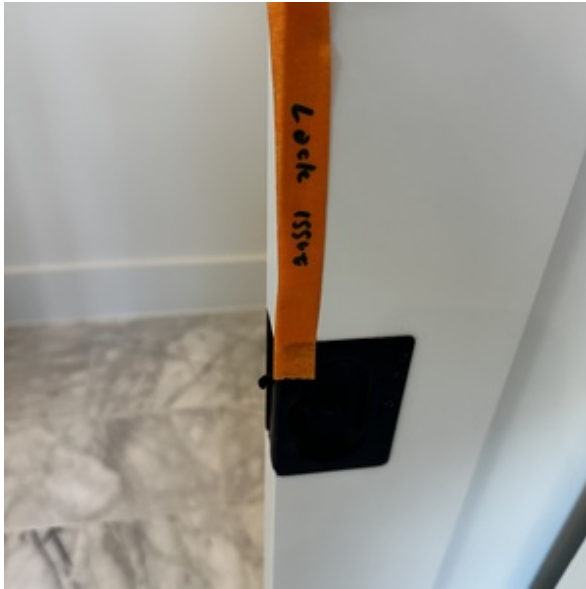
LOCKING ISSUES AT DOORS
