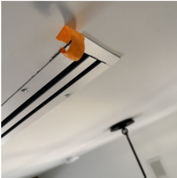
MINOR FLAWS MARKED ON SITE
