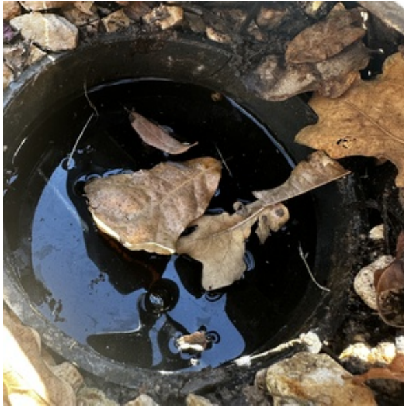
STANDING WATER IN VALVE BOX
