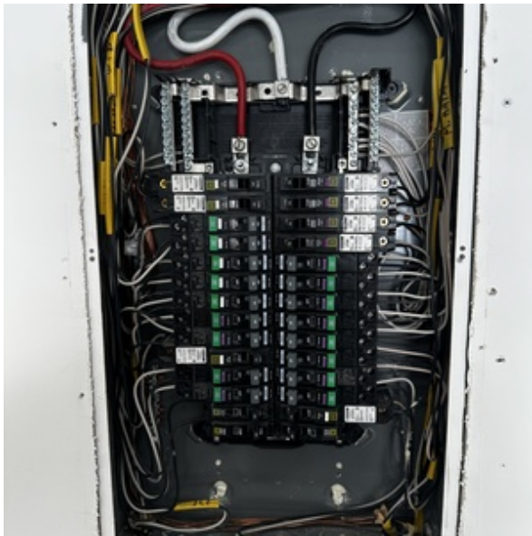
SUB PANEL IN GARAGE
