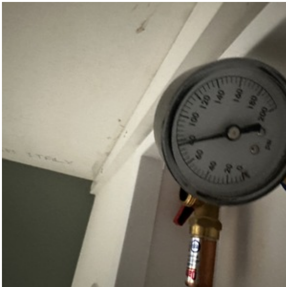
SUPPLY PRESSURE TEST FAILED
