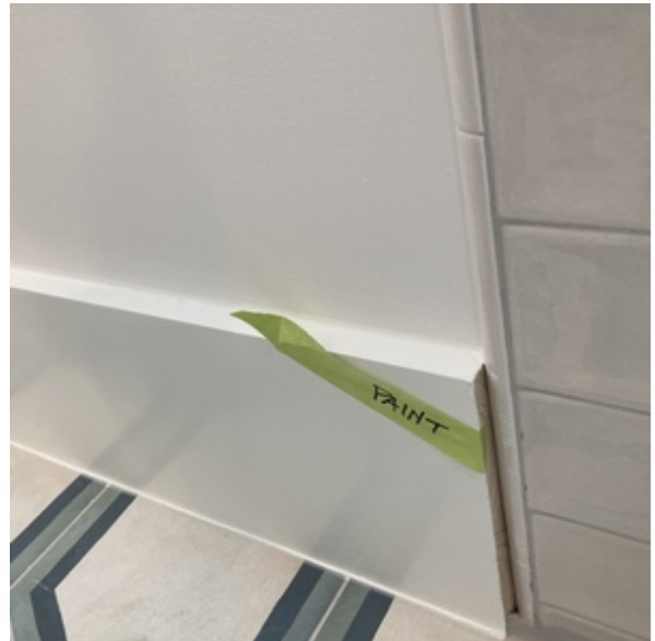
MINOR FLAWS MARKED ON SITE
