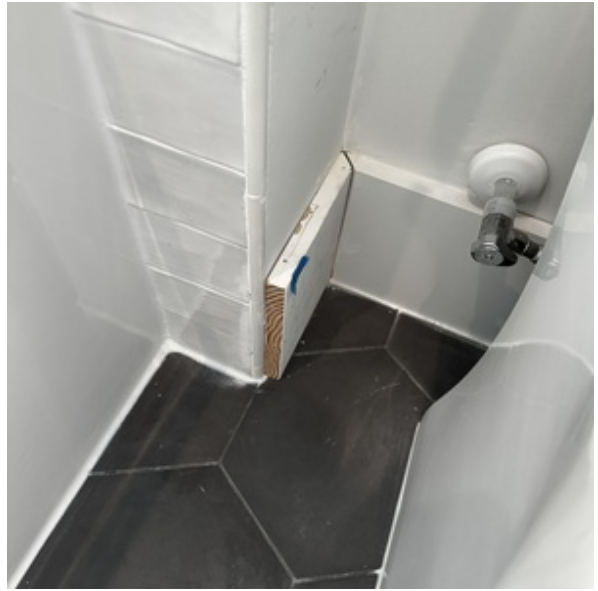
INCOMPLETE TRIM WORK (BATHROOM)
