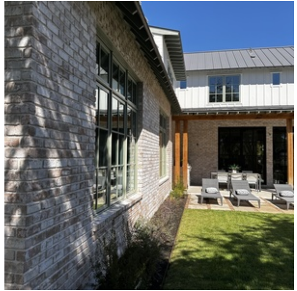
RAIN GUTTERS NOT PROVIDED
