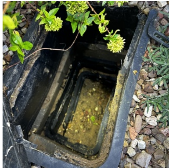
BOX NEAR CLEANOUT - PURPOSE UNKNOWN
