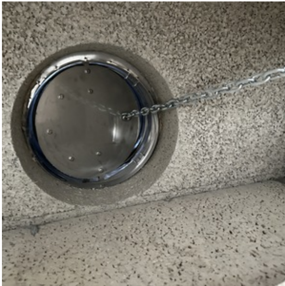
FLUE DAMPER PROVIDED
