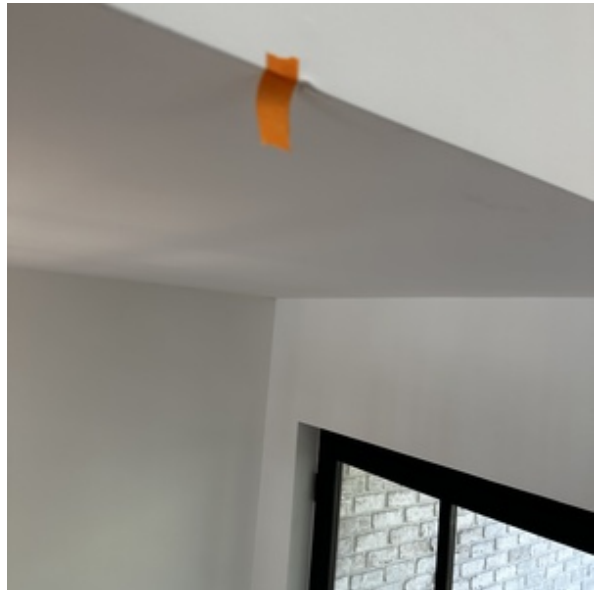
MINOR FLAWS MARKED ON SITE
