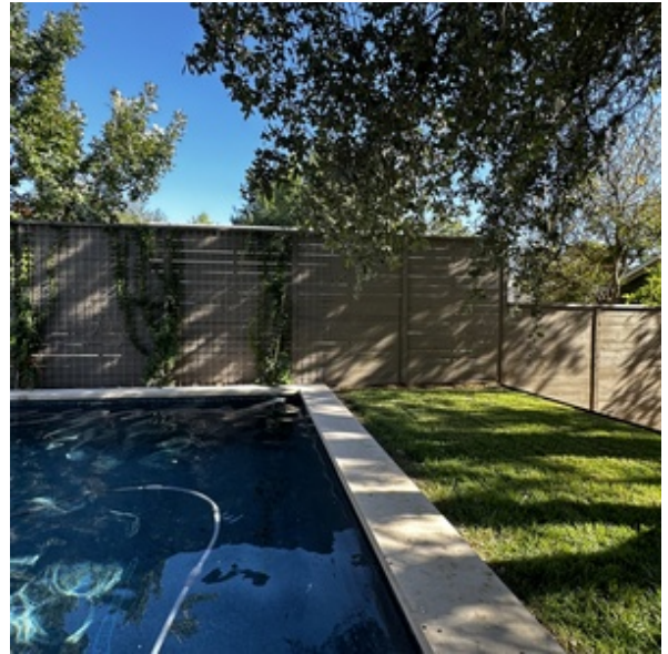
NO SURROUNDING DECKING
