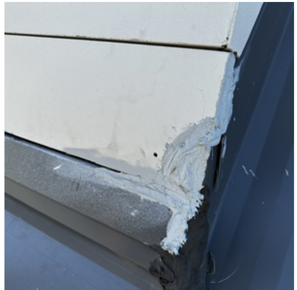
POSSIBLE CAULK DEPENDENT FLASHING
