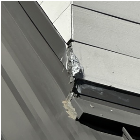
POSSIBLE CAULK DEPENDENT FLASHING
