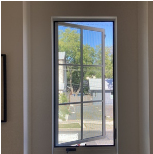
WOOD FRAMED WINDOWS PRESENT
