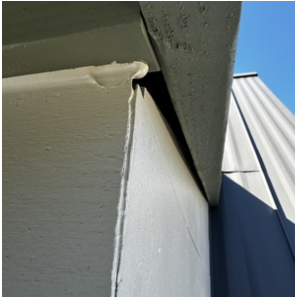
SEAL GAPS AT FASCIA AREAS
