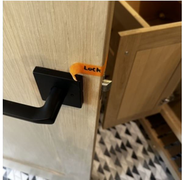
LOCKING ISSUES AT DOORS
