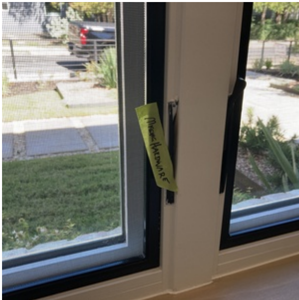
COMMON ISSUES MARKED ON SITE
