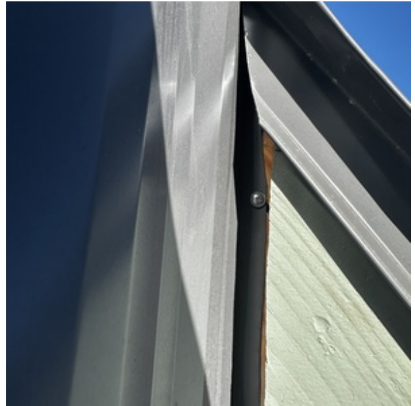
SEAL GAPS AT FASCIA AREAS
