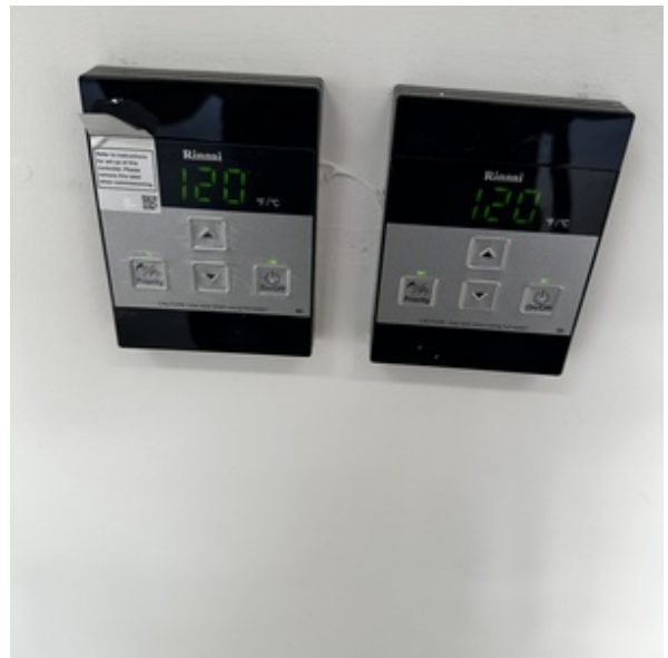
CONTROLS IN GARAGE
