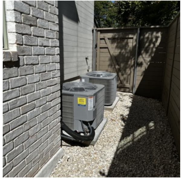
EQUIP. UNDER FLAT ROOF DRAIN POINT
