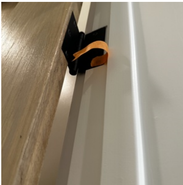
COMMON FLAWS MARKED ON SITE
