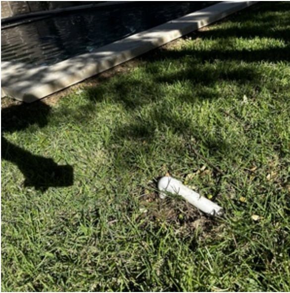
PIPE NEAR POOL: PURPOSE UNKNOWN
