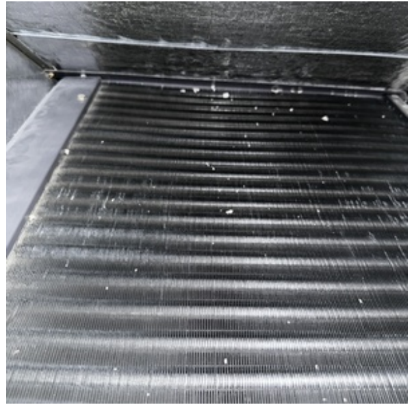
AHU: NO ISSUES DISCOVERED
