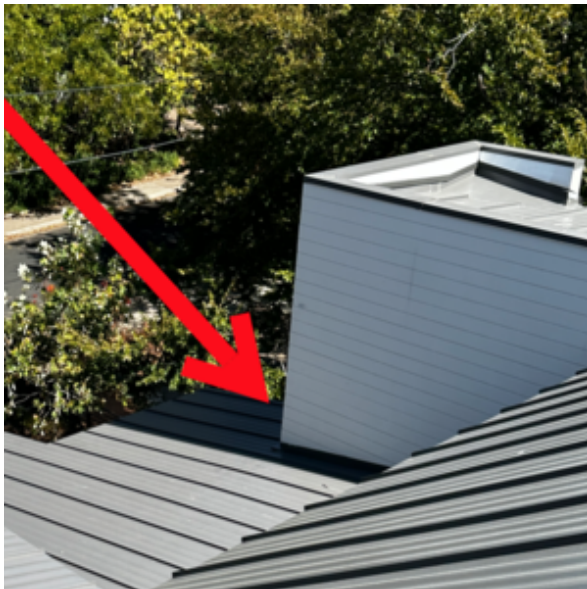
AREA OF GAP/BARRIER FLAW
