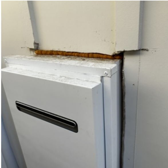
GAP/CUTS SURROUNDING W/H
