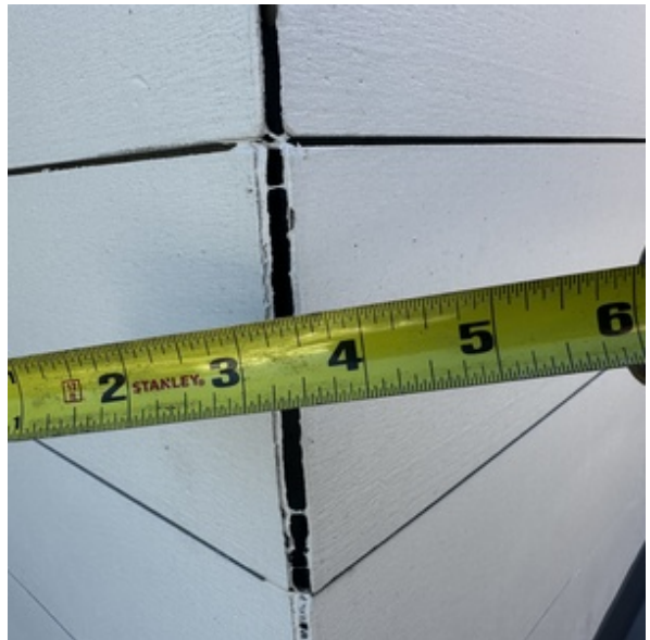
CLADDING GAP NEAR BARRIER FLAW
