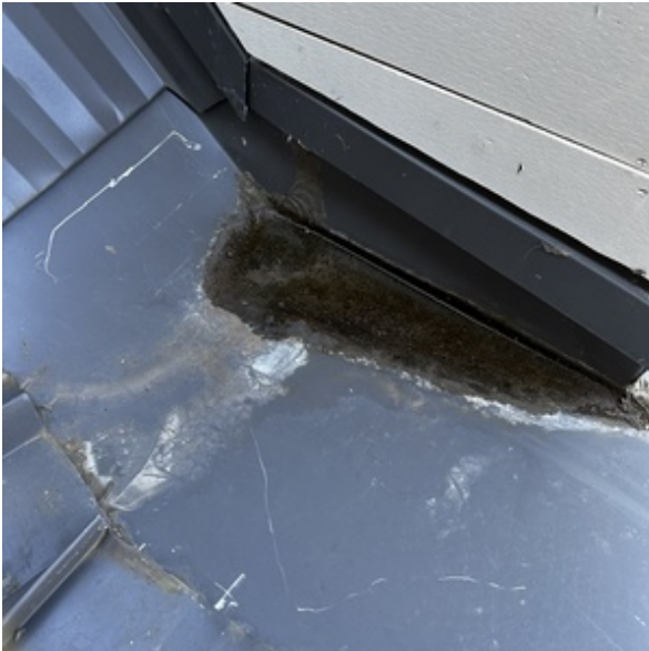
POOLING WATER AT FLASH PAN
