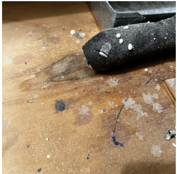
MOISTURE CONCERN NEAR DRAIN
