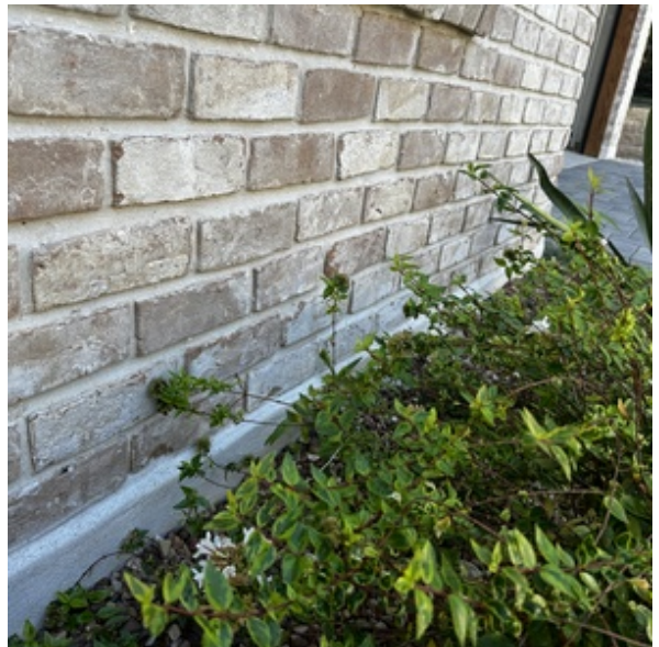
AREA OF MISSING/REDUCED WEEPHOLES
