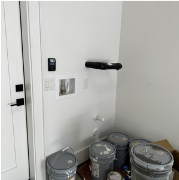
WATER SOFTENER STAGING AREA
