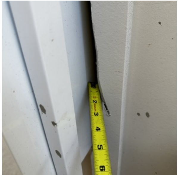
GAP/CUTS SURROUNDING W/H
