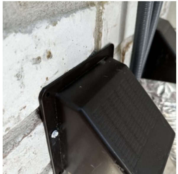
CAULK/SEAL AT HVAC LINE CAP
