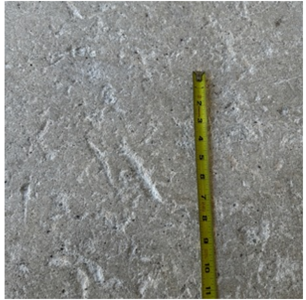
GARAGE SURFACE FLAWS
