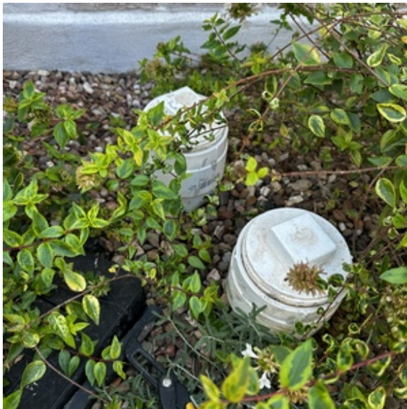
CLEAN OUT RISERS - FRONT YARD
