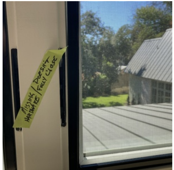
COMMON ISSUES MARKED ON SITE
