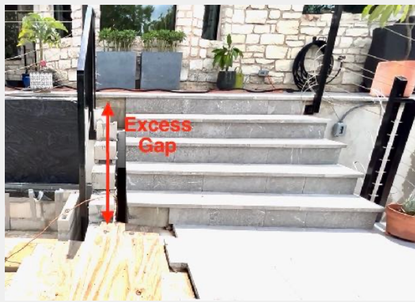
Gap at Stairs
