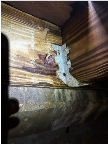
DEFERRED MAINTENANCE AT DECKING
