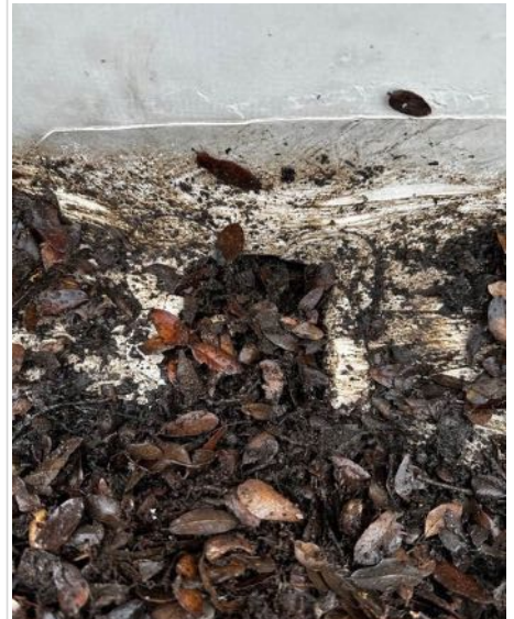
DEBRIS/DRAINAGE ISSUES AT ROOF
