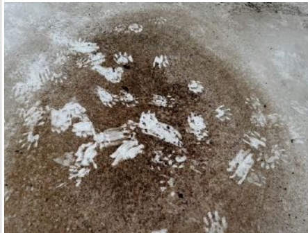
VERMIN ACTIVITY AT ROOF LEVEL
