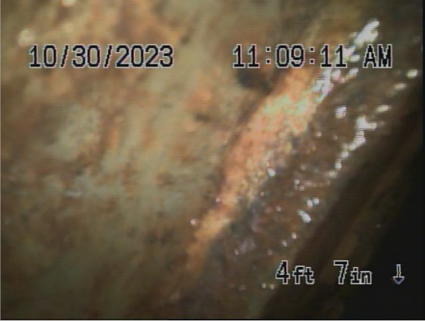
ENTRY FROM CLEAN OUT FAILED, INDICATOR OF CAST IRON NOTED
