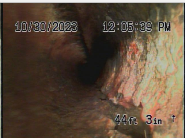
PIPE DAMAGE/FAILURE: 44' FROM V1
