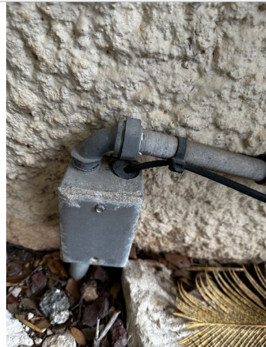
ELECTRICAL SERVICE NEEDS
