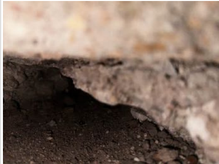
GAPS UNDER EXTERIOR SLAB
