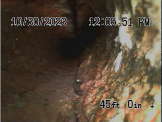
PIPE DAMAGE/FAILURE: 45' FROM V1
