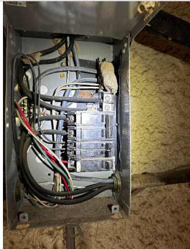
ELECTRICAL SERVICE NEEDS
