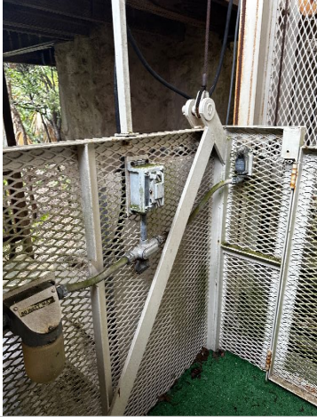
ELEVATOR NOT FUNCTIONAL
