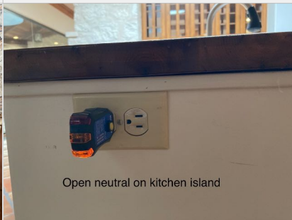
OUTLET WIRING ISSUE
