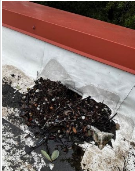
DEBRIS/DRAINAGE ISSUES AT ROOF
