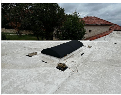
DATED, DAMAGED SKYLIGHTS
