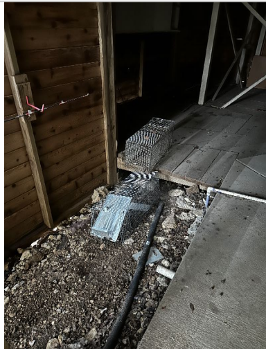
DEFERRED MAINTENANCE AT DECKING
