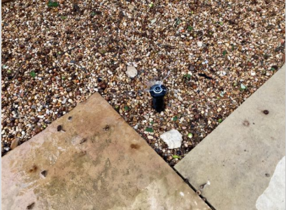
WEAK PRESSURE AT IRRIGATION SYSTEM
