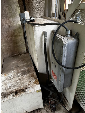
ELEVATOR NOT FUNCTIONAL
