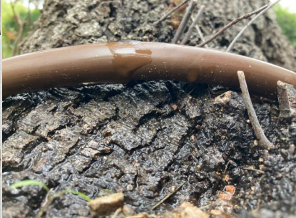
WEAK PRESSURE AT IRRIGATION SYSTEM
