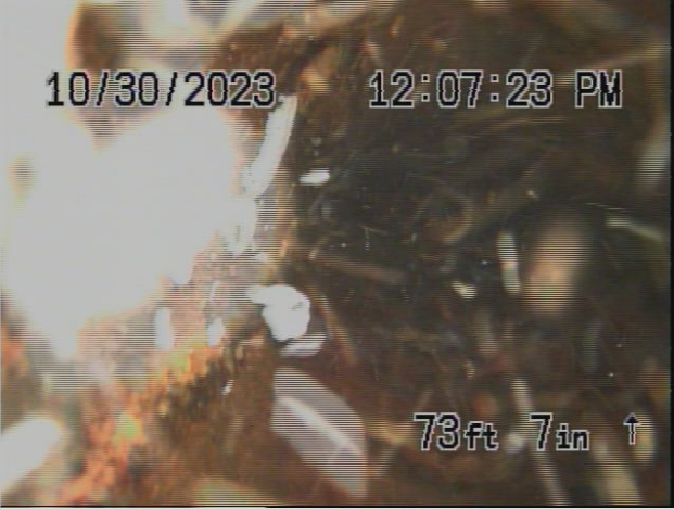
DRAINAGE OBSERVED AT CAST IRON
