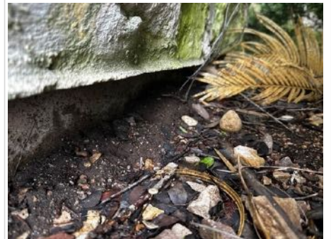
UNSUPPORTED MASONRY WALL
