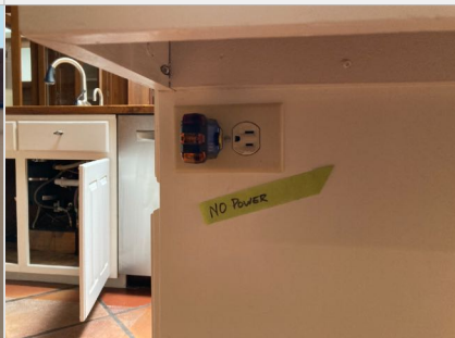
DEAD OUTLETS/FAILED BREAKERS
