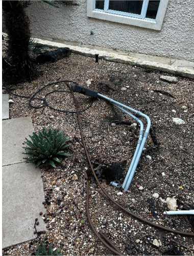
ELECTRICAL SERVICE NEEDS
