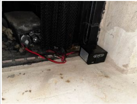
DAMAGED FIREPLACE DEVICES
