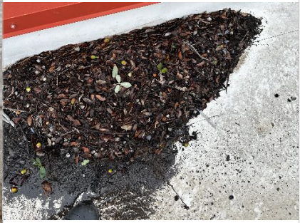
DEBRIS BUILD UP
