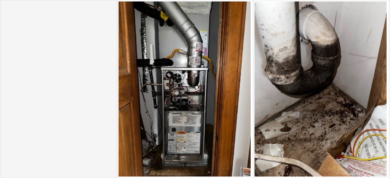
VARIOUS SERVICE, REPAIR, AND UPDATE NEEDS
