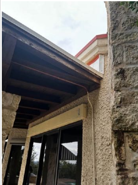
DECK DETERIORATION ISSUES
