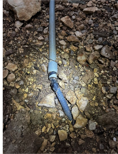
ELECTRICAL SERVICE NEEDS
