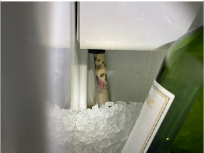
DATED APPLIANCES REQUIRE SERVICING
