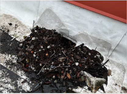
ROOF DRAIN ISSUES
