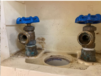
LEAKING LAUNDRY HOOK-UPS
