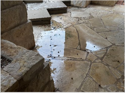
POOLING AT FRONT PORCH
