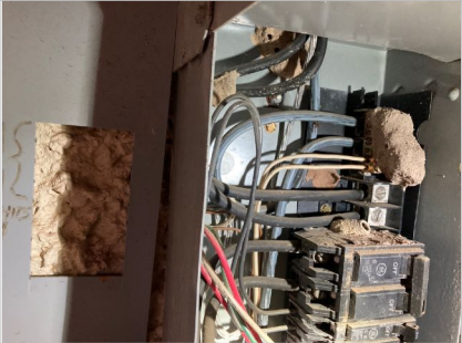
EQUIP. SERVICE NEEDS
