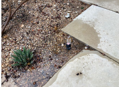
WEAK PRESSURE AT IRRIGATION SYSTEM
