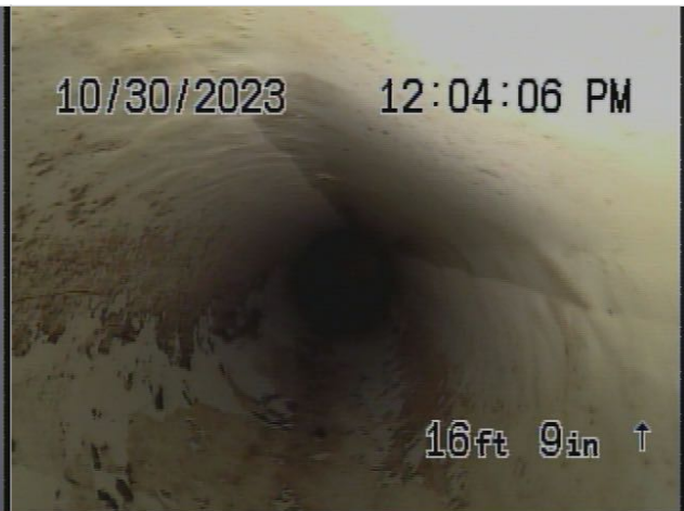
VENT AND PORTION OF DRAIN IS PVC
