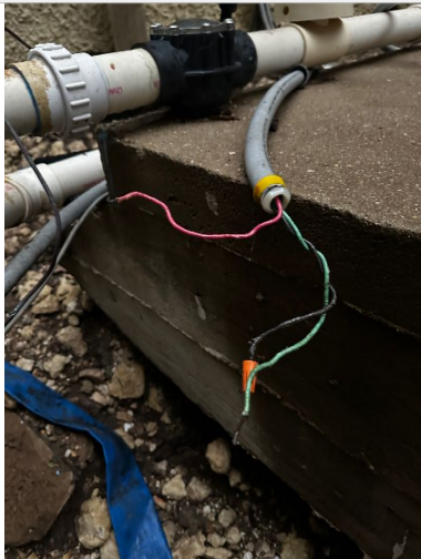
ELECTRICAL SERVICE NEEDS
