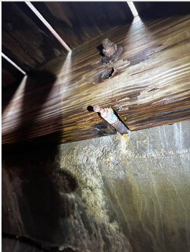
DEFERRED MAINTENANCE AT DECKING
