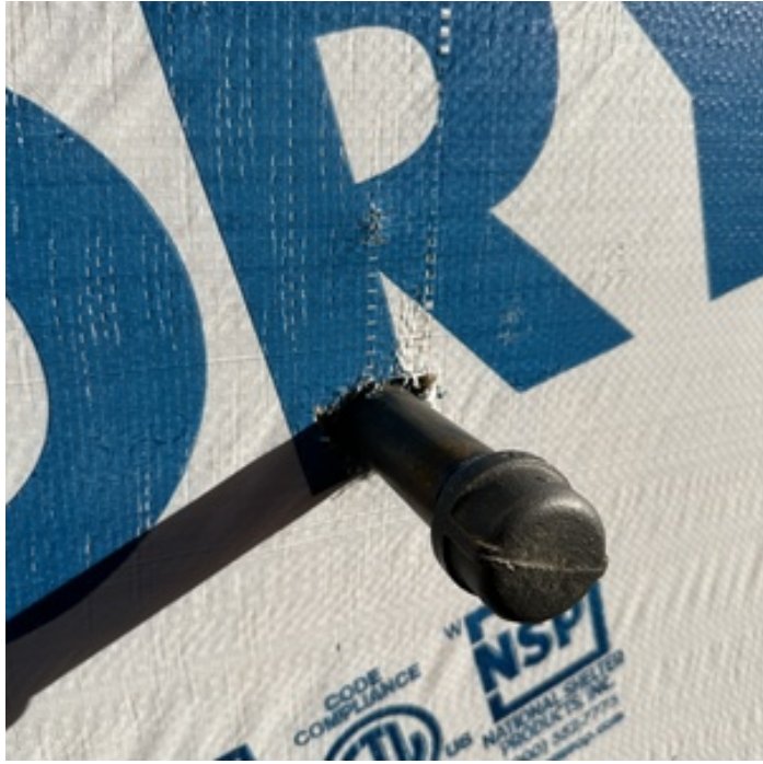
TAPE AT PENETRATIONS
