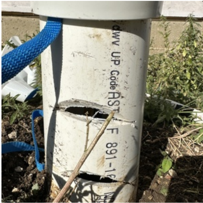
DAMAGED CLEANOUT RISER
