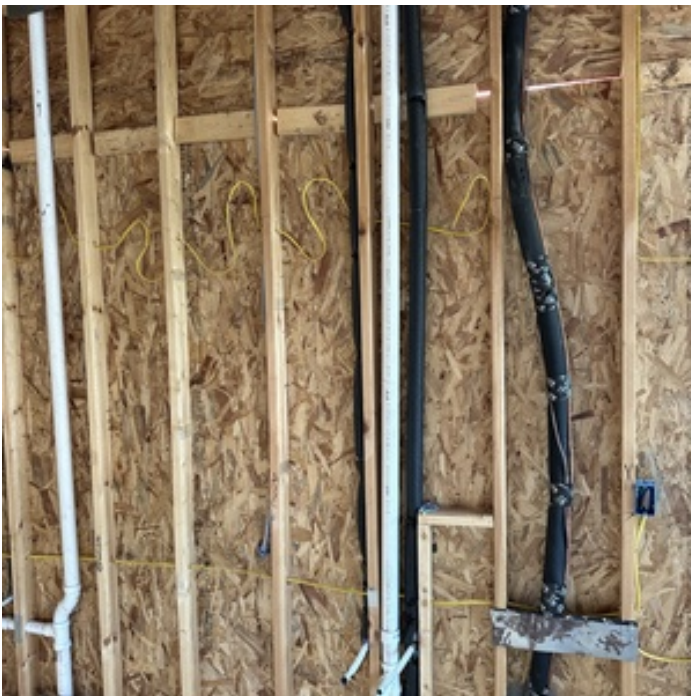
ENSURE INCOMPLETE CIRCUITS FINISHED
