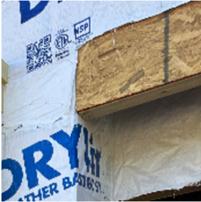
AREAS OF INCOMPLETE BARRIER
