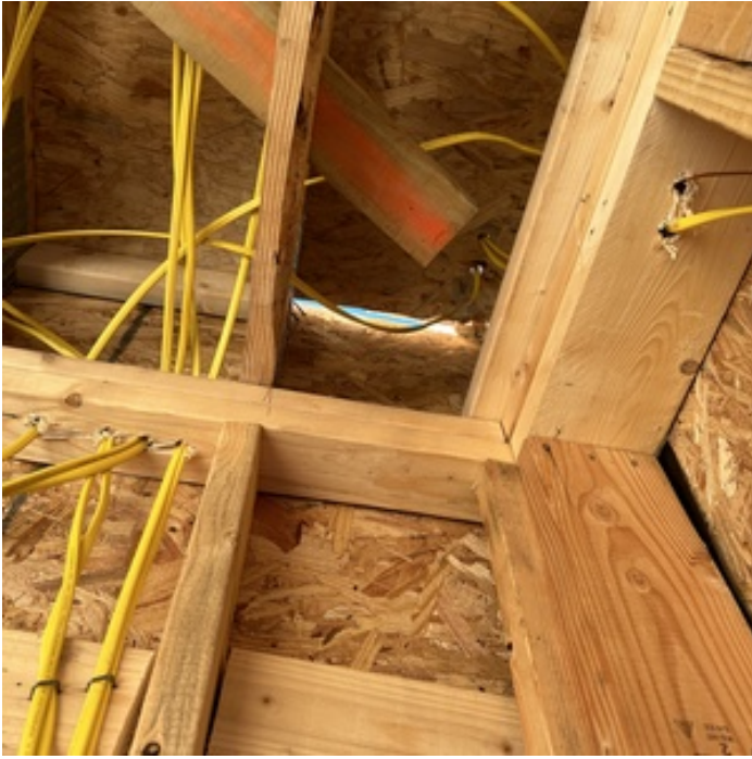
ADDRESS DECKING GAPS
