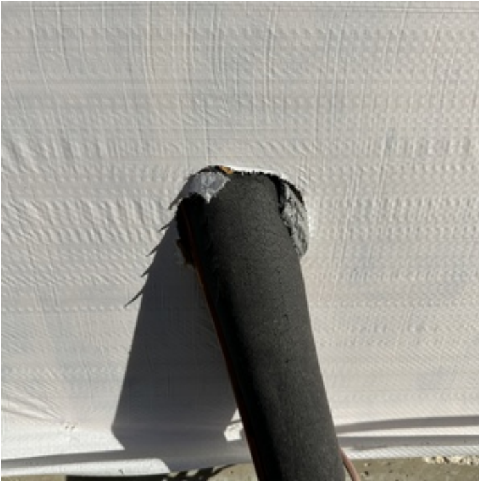
TAPE AT PENETRATIONS
