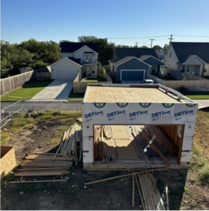
INCOMPLETE FLAT ROOF WORK
