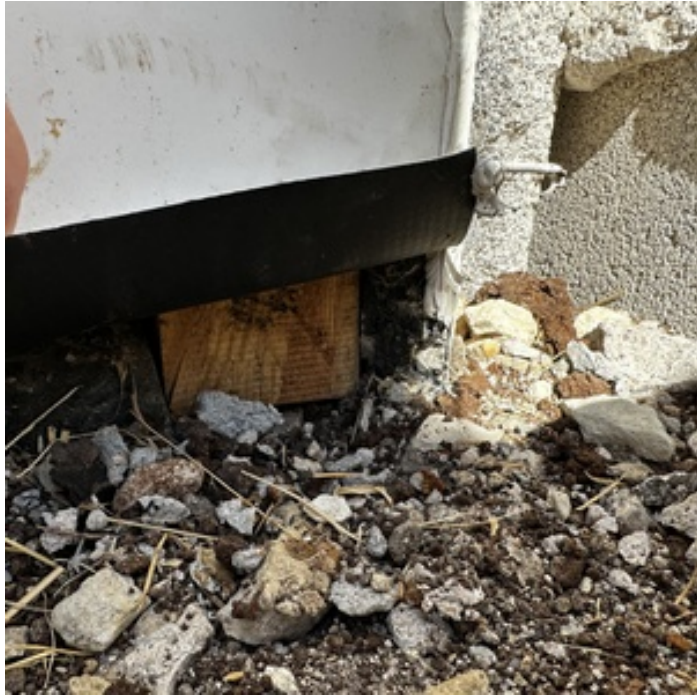
EXPOSED PLYWOOD, LOOSE TPO
