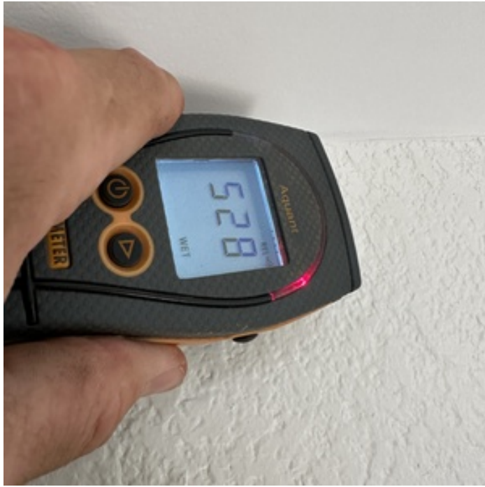
DINING: ELEVATED MOISTURE READINGS
