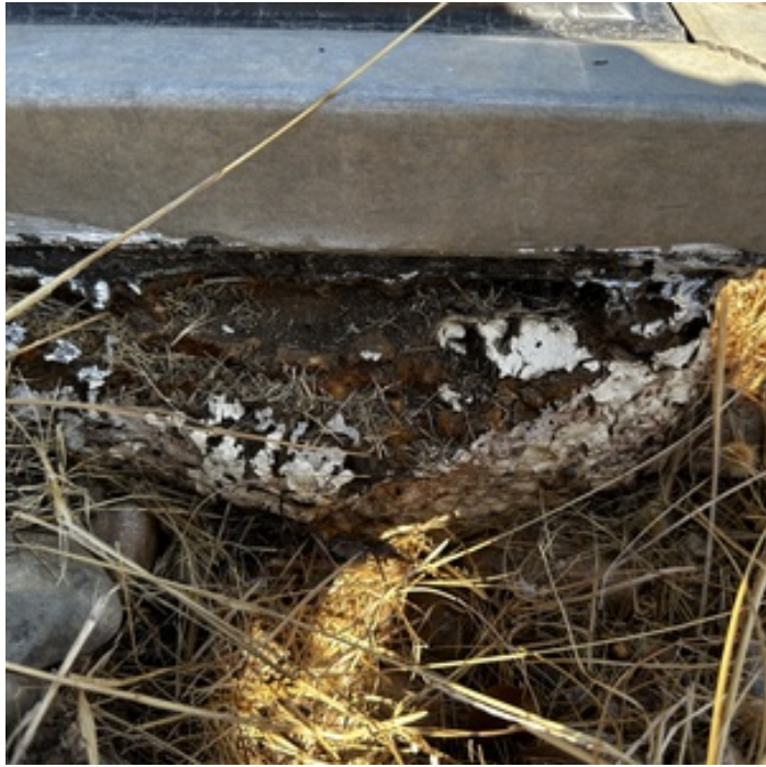
DETERIORATION OF FOAM SURROUNDING
