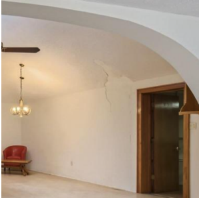
PREVIOUS DAMAGE NEAR HIGH READING
