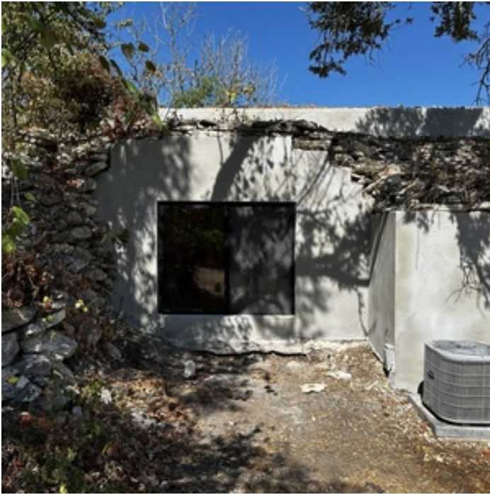
DRAINAGE CONCERN OVER WINDOW
