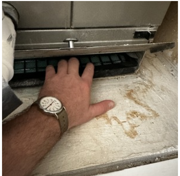
PREVIOUS HVAC LEAK
