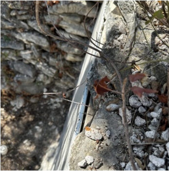
NO UPPER CLADDING FLASHING
