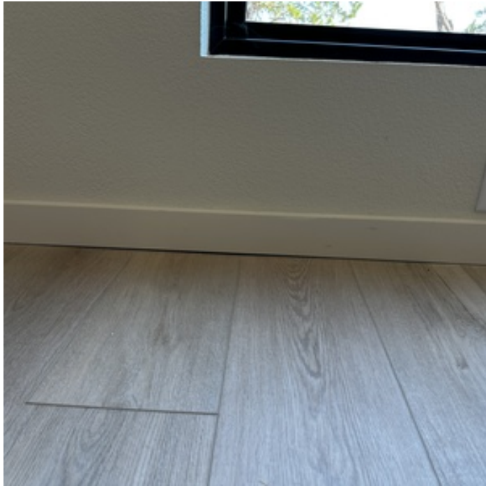
AREAS OF UNEVEN FLOOR SURFACES
