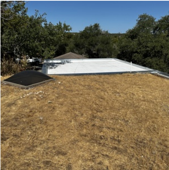
UNIQUE DRAINAGE NEEDS AT ROOF
