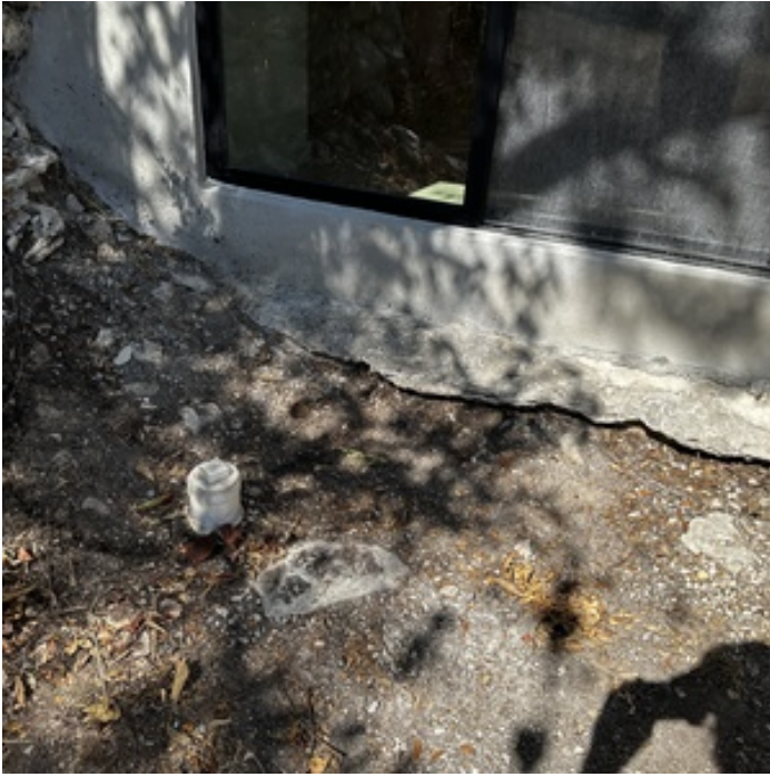
DRAINAGE ISSUE NEAR LEFT WALL
