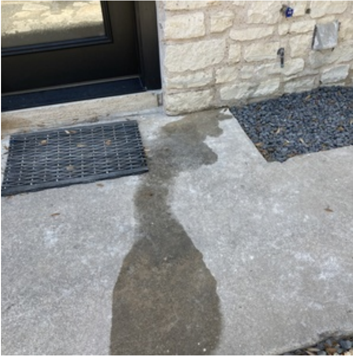
LEAK OVER LAUNDRY/NEAR MAIN ENTRY
