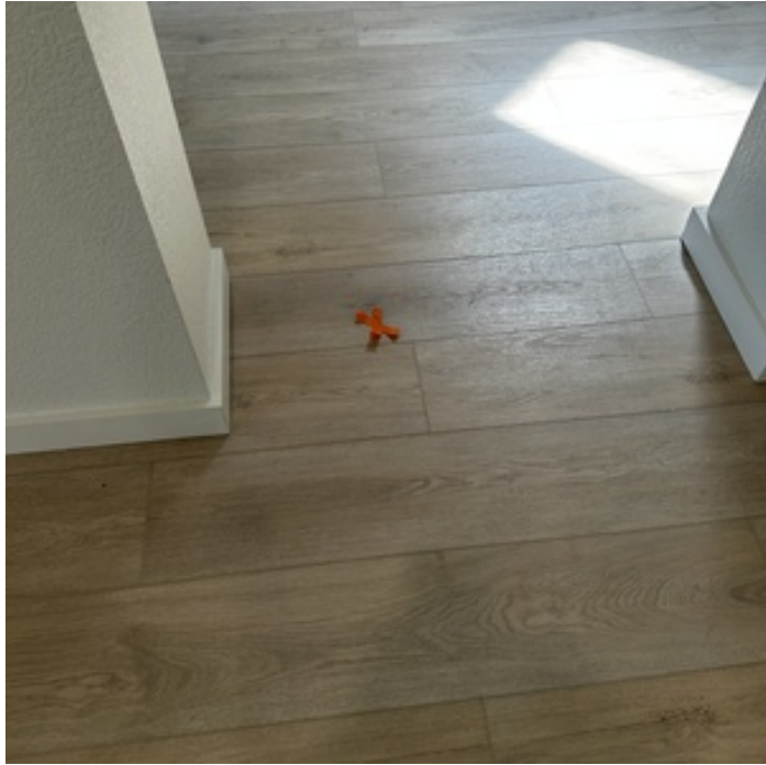
HOLLOW SPOT IN FLOORING
