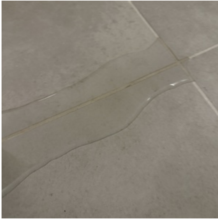
LEAK AT BEDROOM SINK
