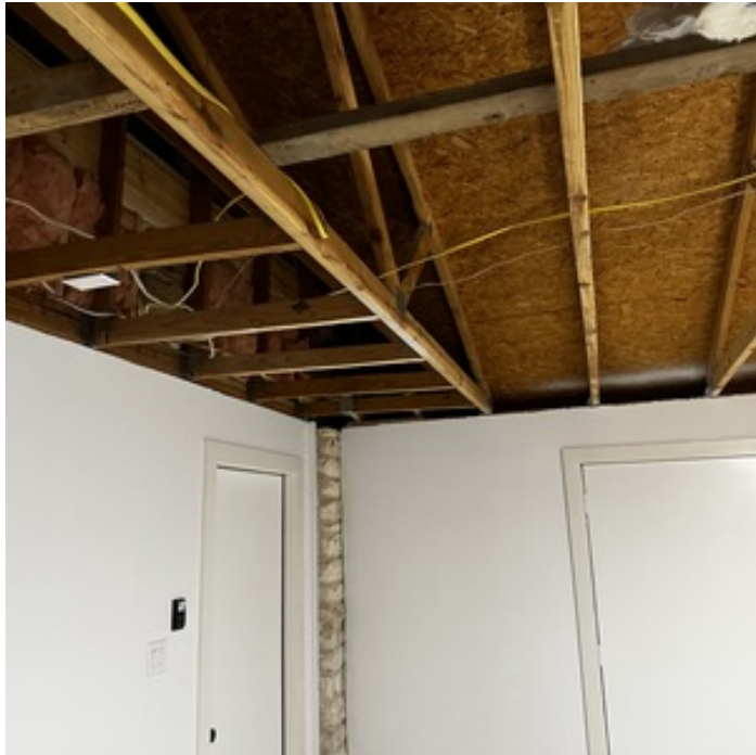
GARAGE: MISSING FIREWALLS
