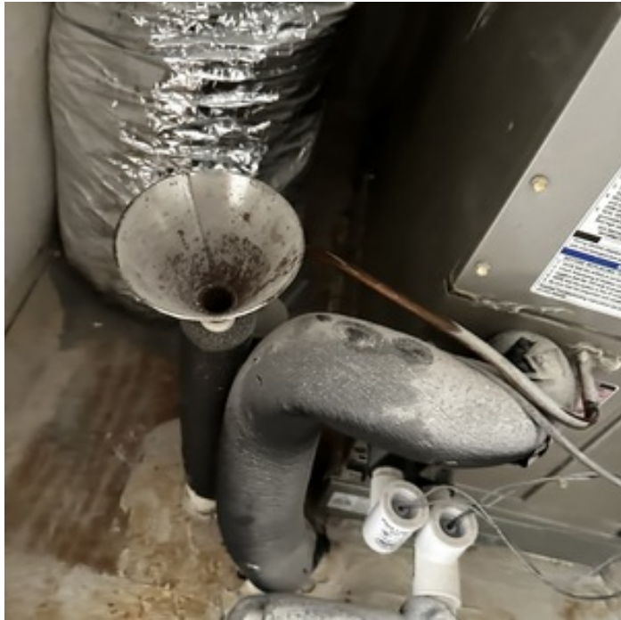
MYLAR FLEX DUCTING OBSERVED
