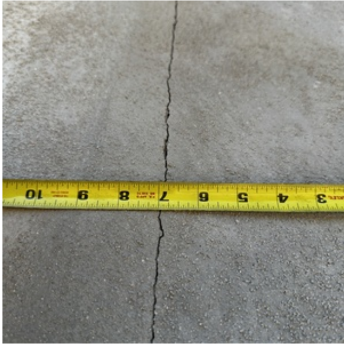
CRACKS AT RECENTLY INSTALLED CLADDING
