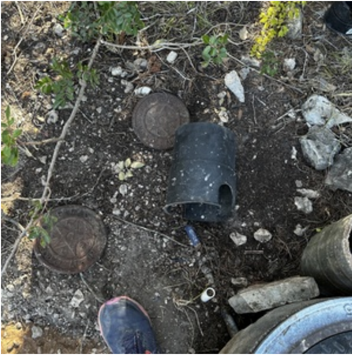
WATER METER RIGHT OF BLDG.
