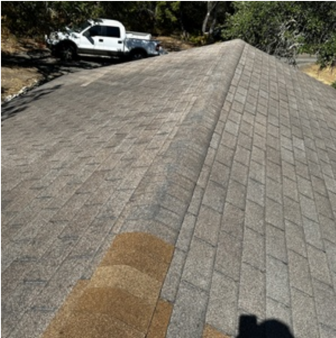
REMAINING SHINGLES IN POOR CONDITION
