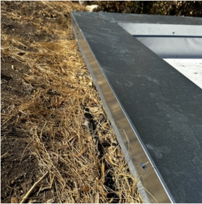
CONCERNS AT ROOF TRANSITION (TESTED)
