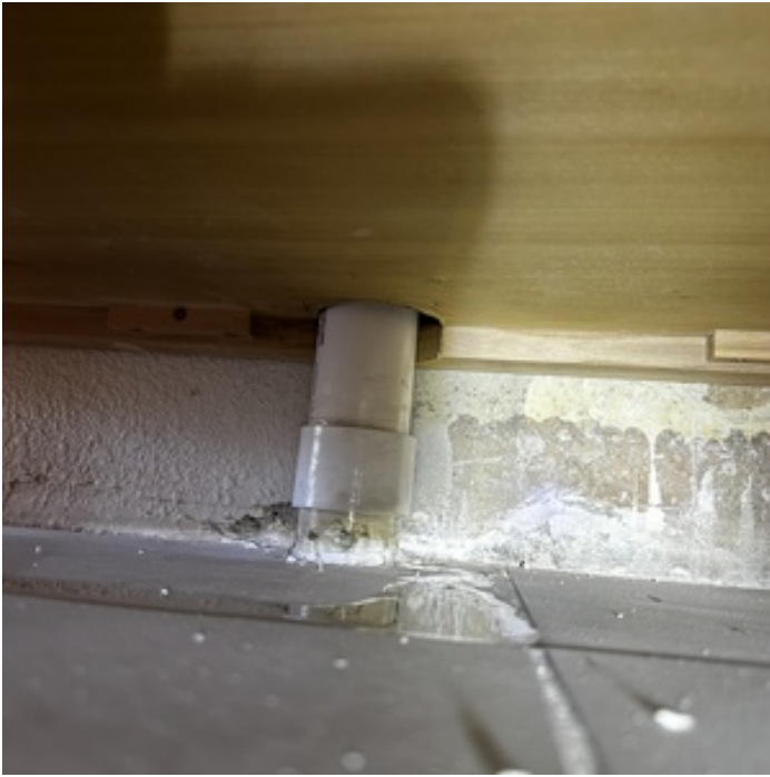
LEAK AT BEDROOM SINK
