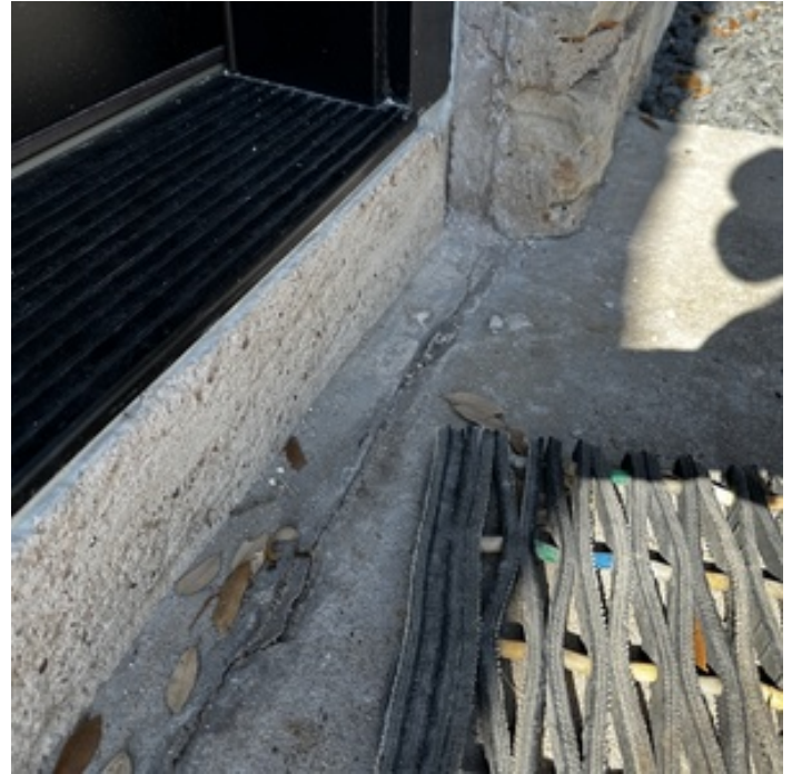
CRACKS AT ENTRY PORCH/LANDING
