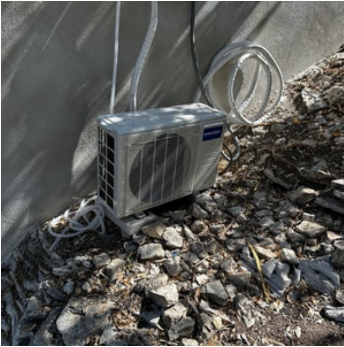
INSTALLATION AND FUNCTIONALITY ISSUES
