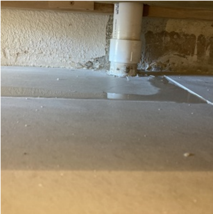
LEAK UNDER BATHROOM SINK
