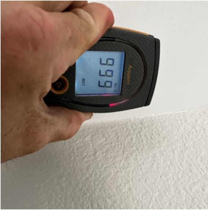
DINING: ELEVATED MOISTURE READINGS
