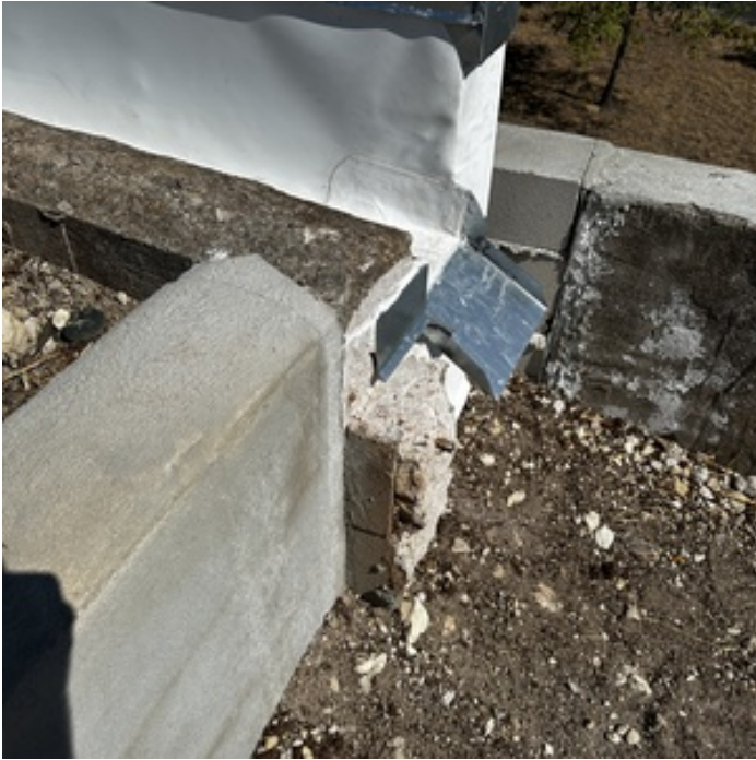
ROOF INTERSECTION CONCERNS
