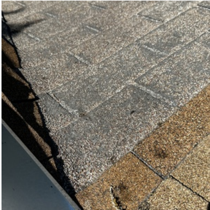
REMAINING SHINGLES IN POOR CONDITION
