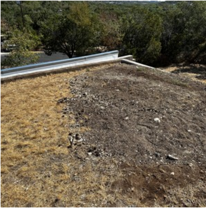
AREA OF PREVIOUS REPAIR
