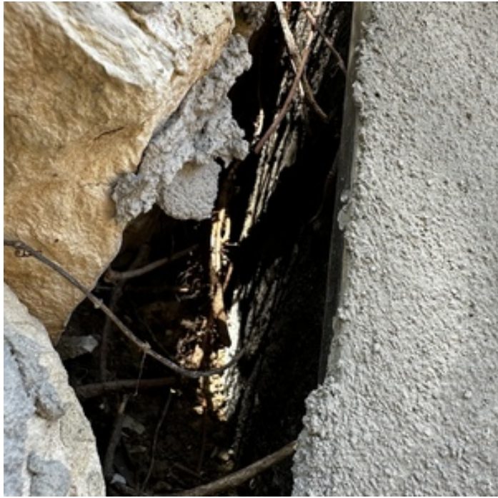
ATYPICAL DRAINAGE POINT AT STONE/CLADDING
