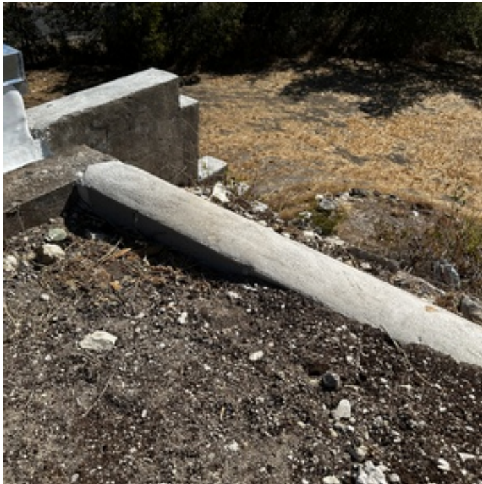
DRAINAGE PATH CONCERNS
