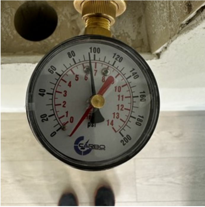
ELEVATED WATER PRESSURE
