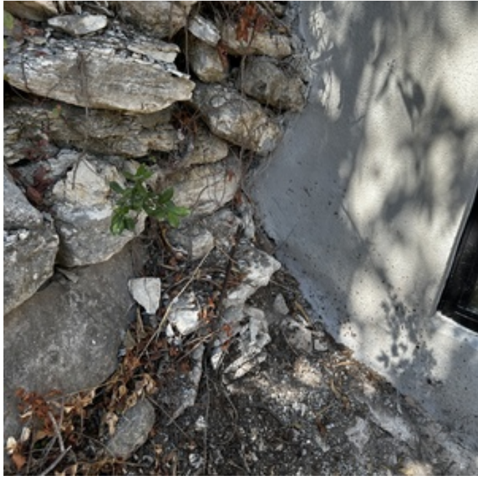
LOOSE DRY STACK ABUTTING WALLS
