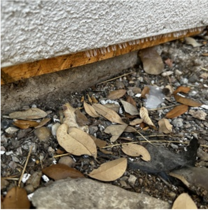
EXPOSED PLYWOOD UNDER STUCCO
