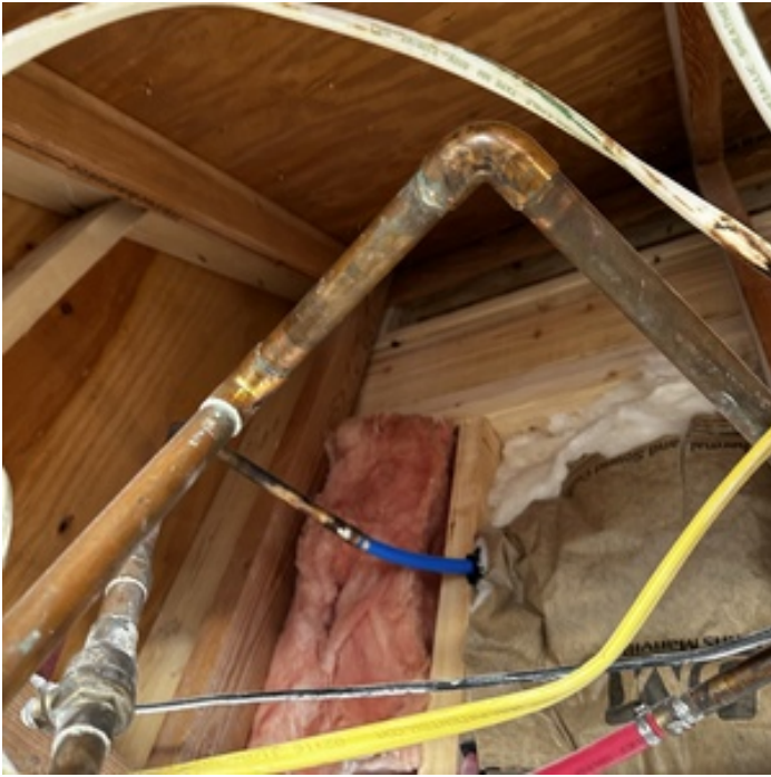
ATYPICAL PIPE CONFIGURATION
