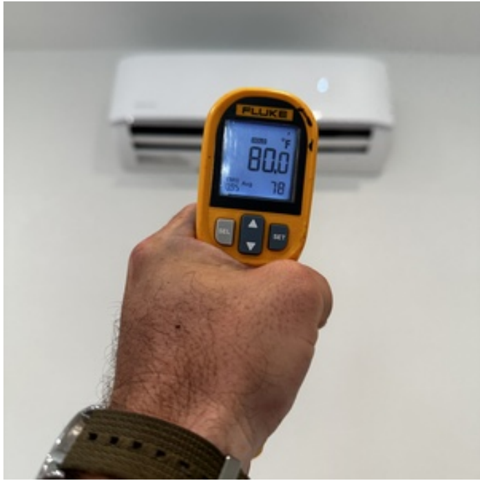
MINI-SPLIT FAILED TO COOL
