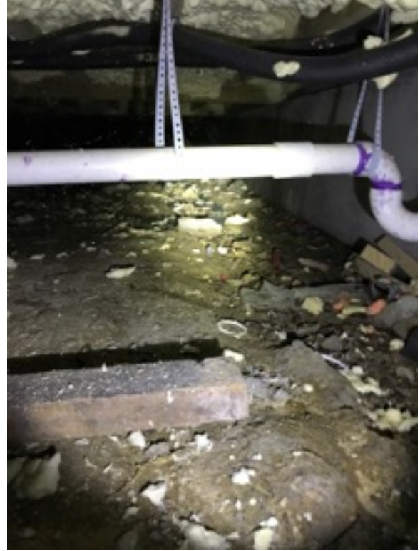
EXCESS MOISTURE AT STEM WALL
