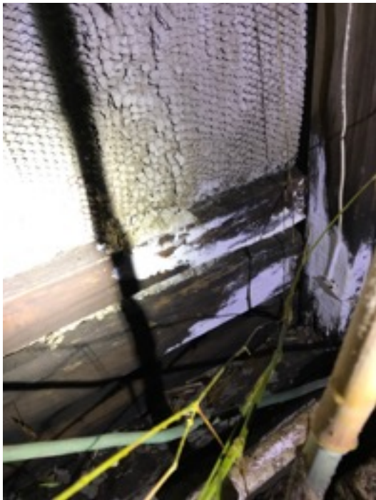
SUSPECT MOLD/FUNGAL GROWTH
