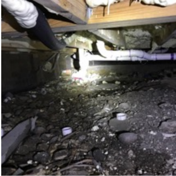
EXCESS MOISTURE AT BACK CORNER
