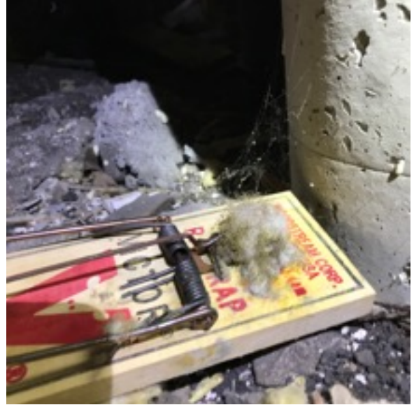
MOLD/FUNGAL GROWTH AT TRAPS
