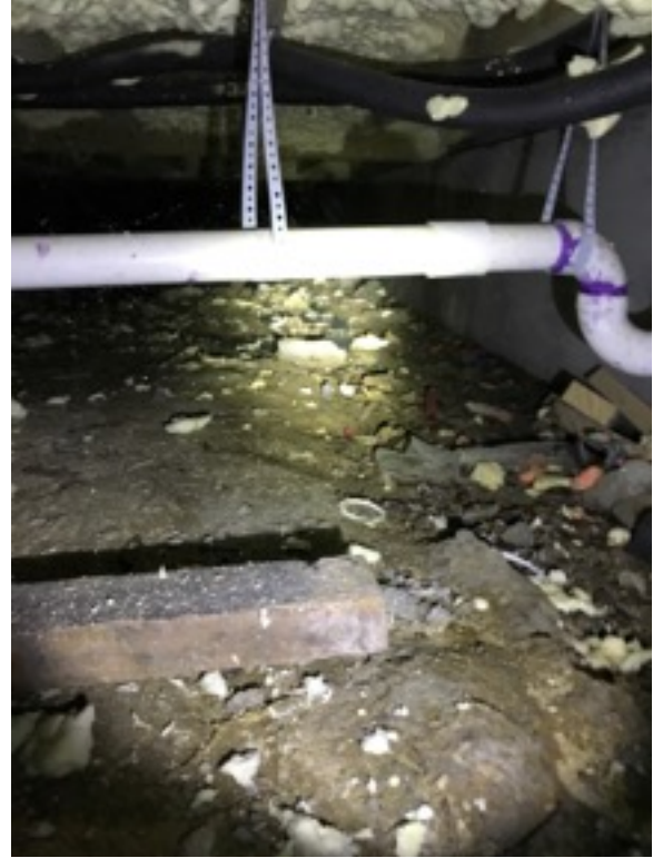
EXCESS MOISTURE AT STEM WALL
