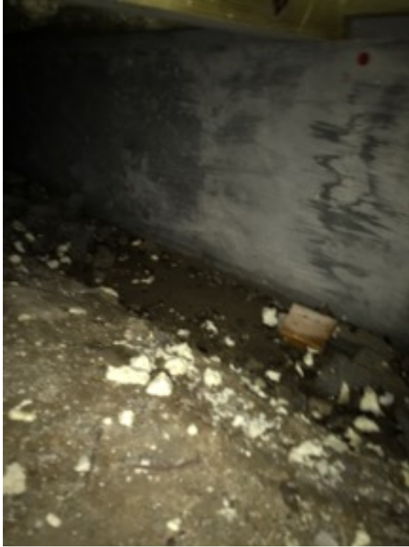
EXCESS MOISTURE AT STEM WALL
